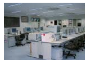
Central monitoring room
