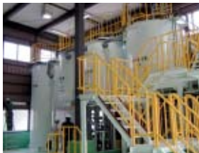
Newly installed hydrofluoric acid treatment system
